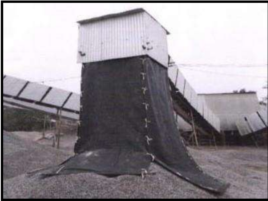
Figure-2: Chute from top of discharge point
